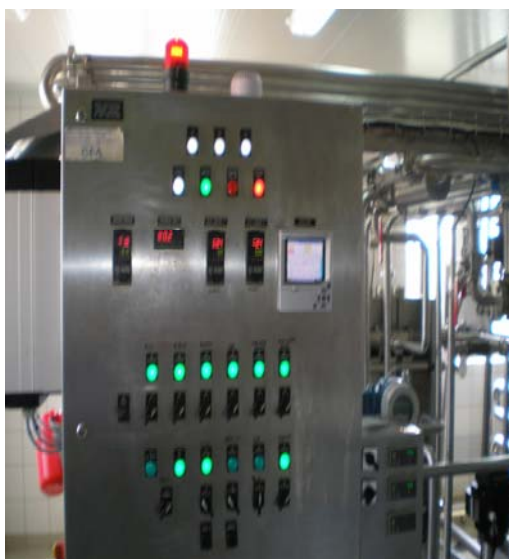
Photo 1. a) Old pasteurizer. b) Automation of pasteurization process
